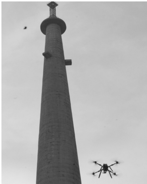
Fig. 17. Structural damage assessment by UAV.
